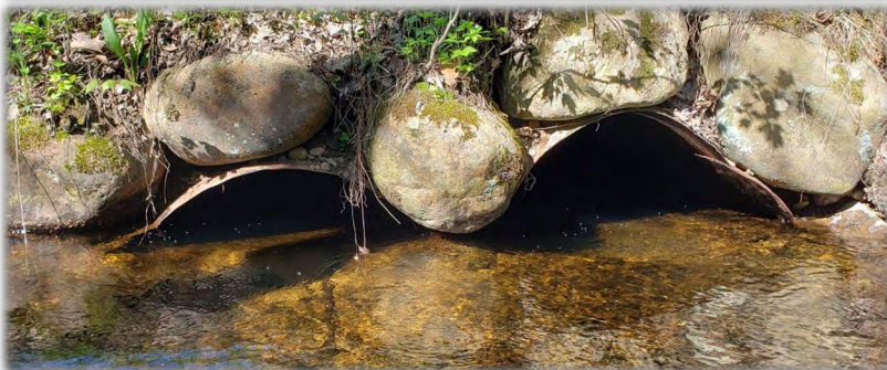
Two of four failing culverts at the output of Rocky Pond in Loudon/Canterbury, before and after the culvert was replaced, thanks to the help of one Conservation Mooseplate Grant completed this past year.
